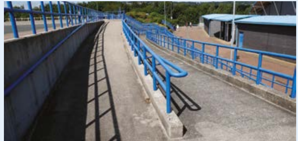
Figure 5 Ramp leading from St Andrew's Upper Level car park to the Magic Rock Stand
